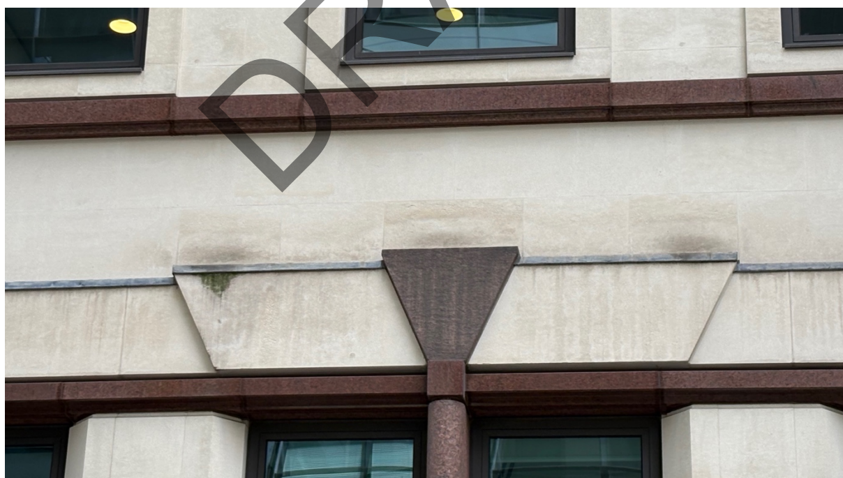
Photograph 14 – Localised damp and algae staining to the original stonework.
